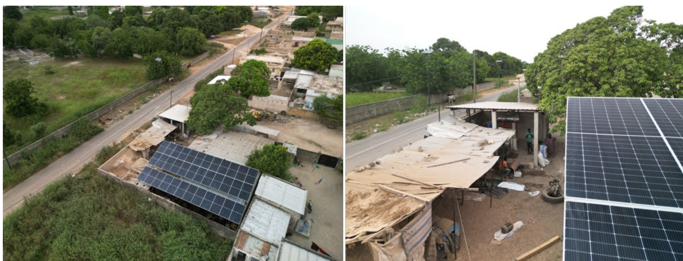
Figure 1: Aerial view of the solar installation at Yaye Aïssatou oil mill.
