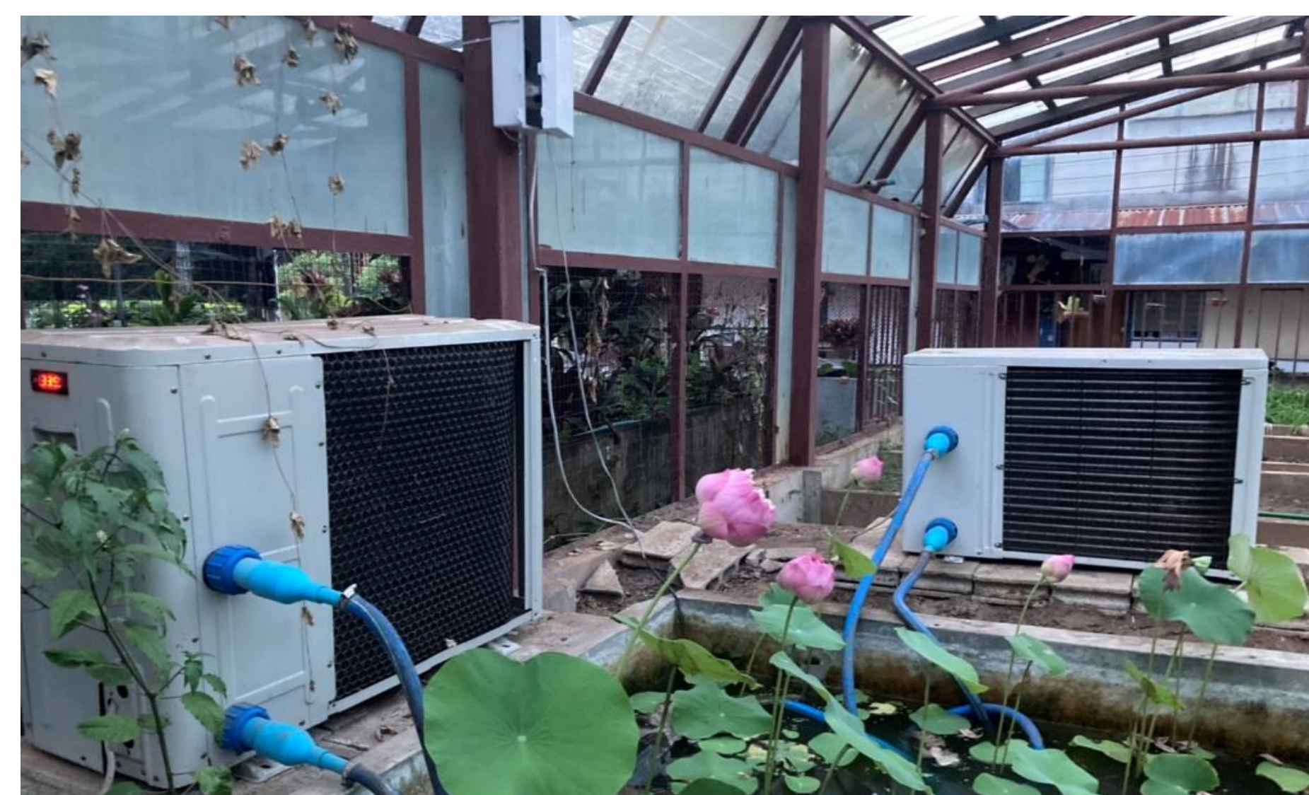
Fig. 1: Cooling unit for controlling the water temperature as a treatment
