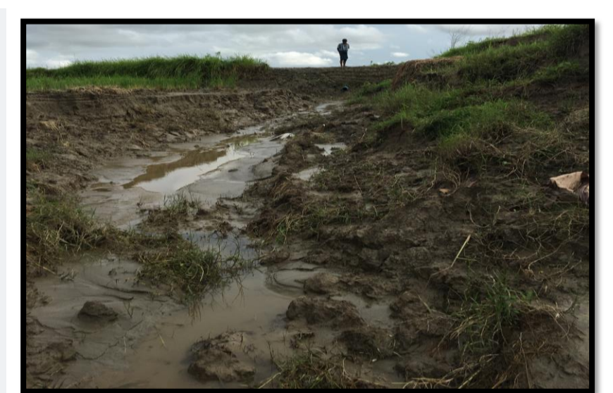
Figure 6: Damage of drainage canal due to erosion
